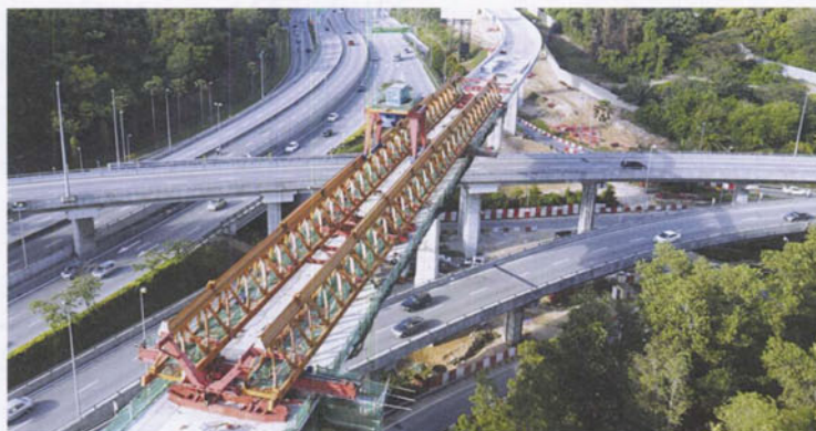
SunCon, undertaking an MRT package, remains confident of securing more projects locally and abroad
